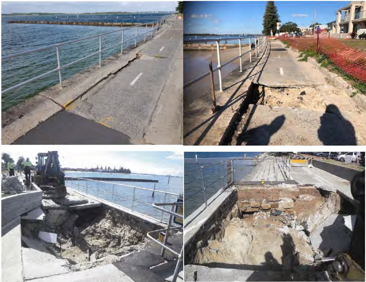
Figure 2-4: Damage to the existing footpath due to loss of backfill from behind the seawall
