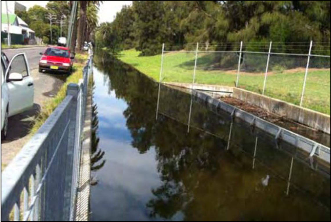
Figure 2-4 Trash rack on Bay Street (near Byrnes Street)
