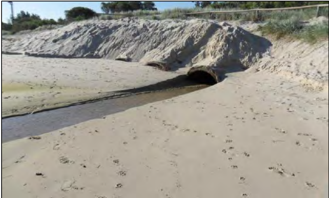
Figure 1-6 Blocked Livingstone Avenue Drain
