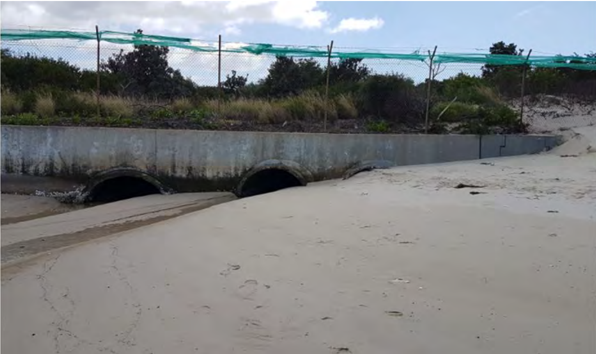
Figure 3.1: Triple pipe outlet near Mill Stream lookout parking bay
