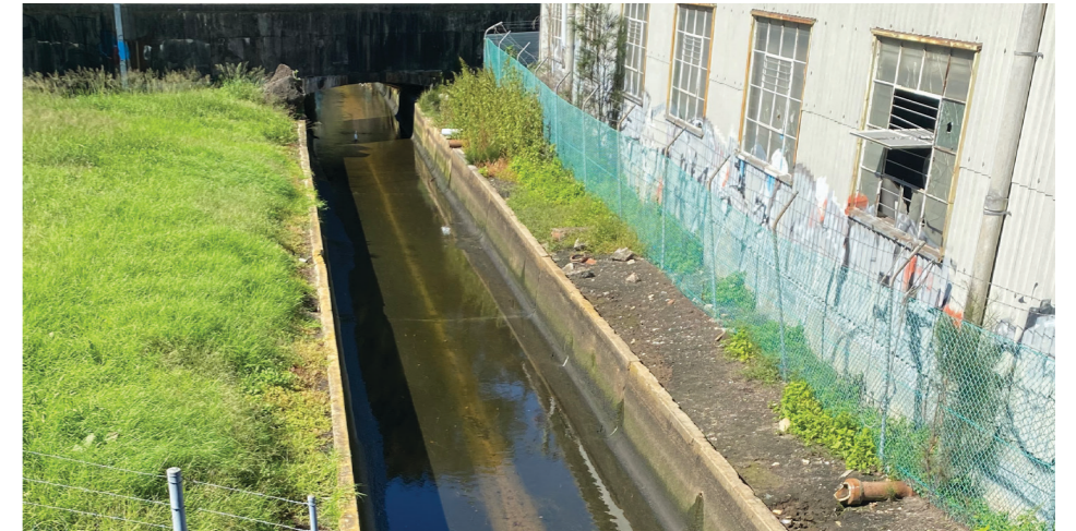
Southern and Western Suburbs Ocean Outfall Sewer (SWOOS), Botany
