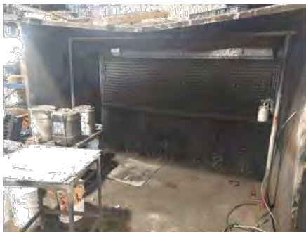
Photo 21. View of the painting cabinet.
