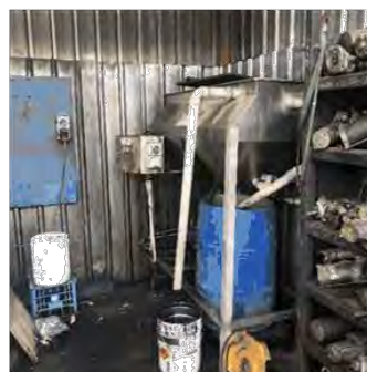
Photo 8. View of the oil / water separator unit.
