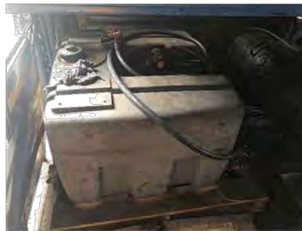
Photo 24. View of the diesel storage tank.
