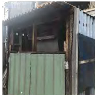
Photo 22. Exhauster system of painting cabinet.
