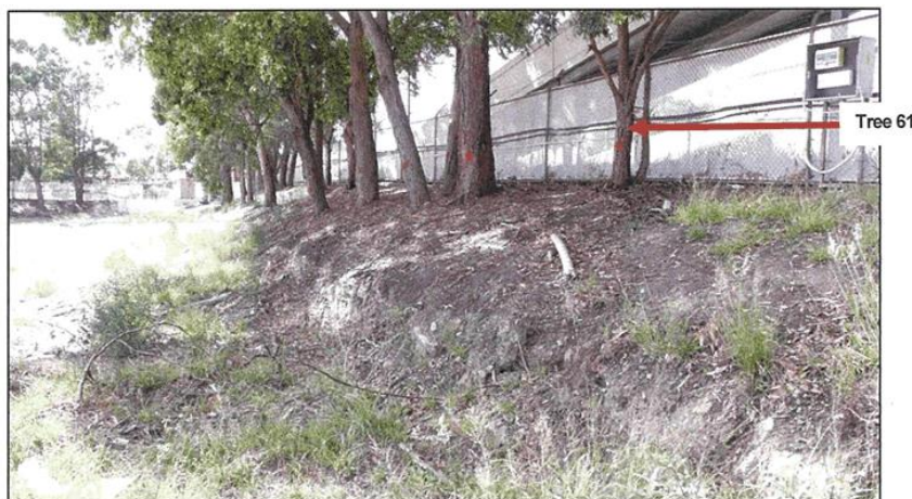
Photo A: Tree 61 to be retained along Westfield Drive frontage. Demolition of the former Carpark included some bulk earthworks and some root damage.
