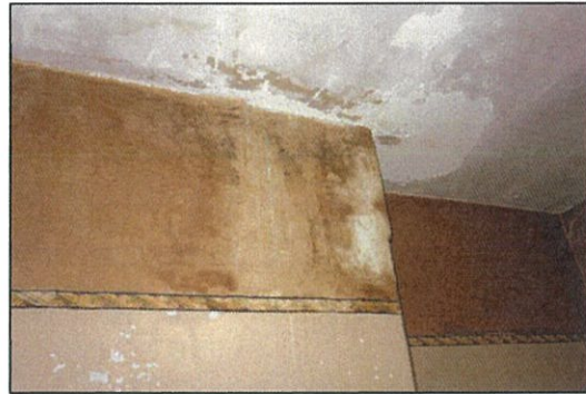
Figure 39. View to wallpapered frieze, Lounge Room. Note evidence of damp damage.
