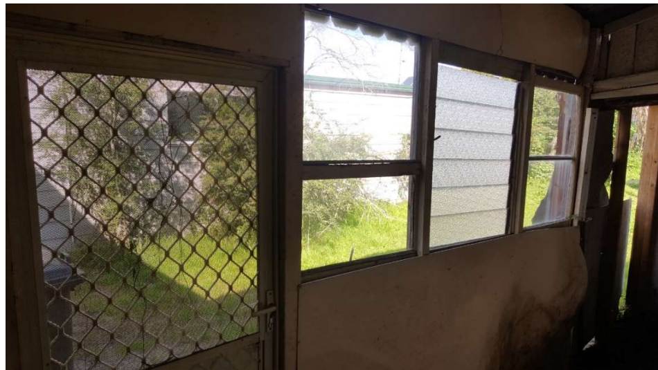
Figure 17 - Later fibro additions to rear of existing house enclosing covered access to kitchen and bathroom, proposed to be demolished.
