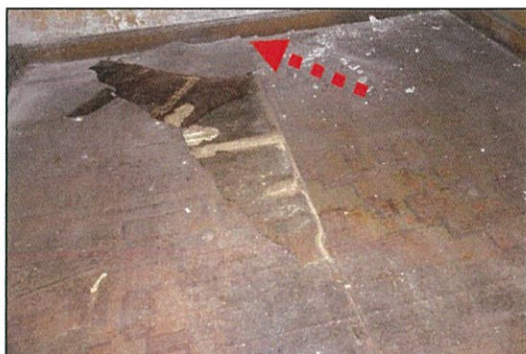
Figure 44. View to linoleum floor covering, Bed 1. Note gap between floor and wall, indicated by the red arrow.
