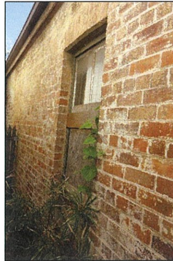
Figure 31. View to W4. Note glazing is missing from the bottom sash, which is currently boarded up.
