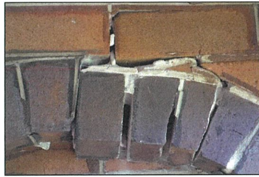
Figure 17. View to dislodged and shifted dark brick trim to relieving arch of verandah blade wall.
