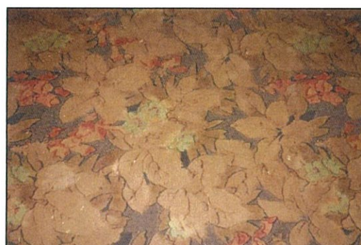
Figure 43. Close-up view to wall paper, Living Room. Faded detail and damp damage observed.
