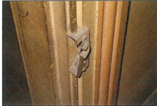
Figure 48. Close-up of damaged door latch, Lounge room.
