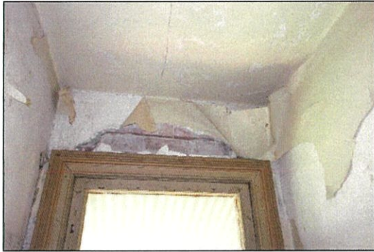
Figure 36. View to peeling plaster and wallpaper as well as exposed brick above main entry door.
