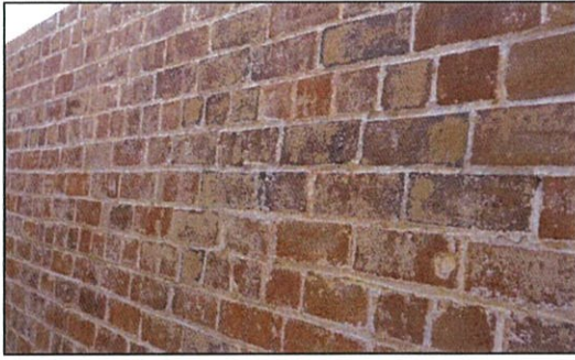
Figure 20. Courser brickwork to side walls, eastern elevation. Note flaked paint coat and spalling.
