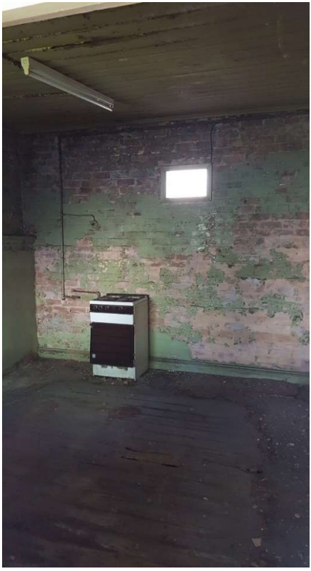
Figure 19 - The kitchen at the rear of the house which is proposed to be demolished.
