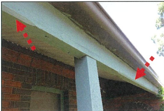
Figure 6. Close-up of painted timber post and verandah beam. Note stop chamfered detail, indicated by the red arrow.
