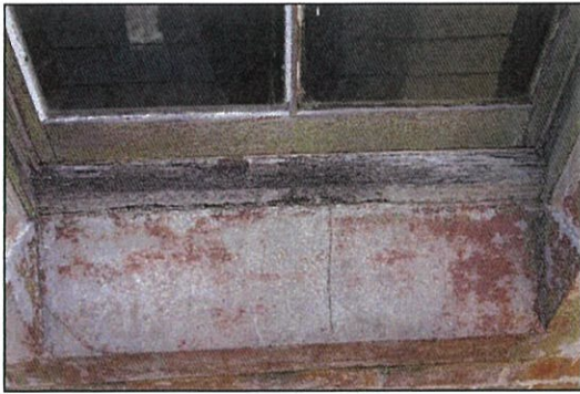
Figure 30. Close-up of W3. Note faded rendered sill. Unseen is a broken window plane to upper sash.
