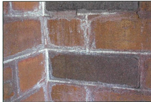
Figure 19. Close-up view of efflorescence, façade.
