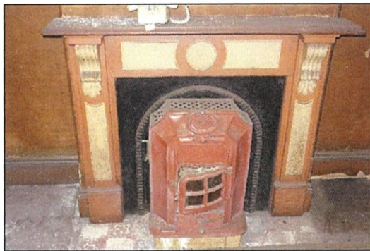
Figure 53. Close-up of fireplace and mantle-piece with cast-iron gas heater and chimney breast, Living room. Note colours to fire-place frame, likely original.
