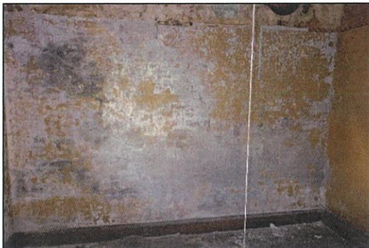
Figure 38. View to cracked and flaked wall paper, Bedroom 1.
