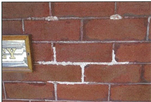
Figure 18. Close-up view of unmatching mortar, façade.
