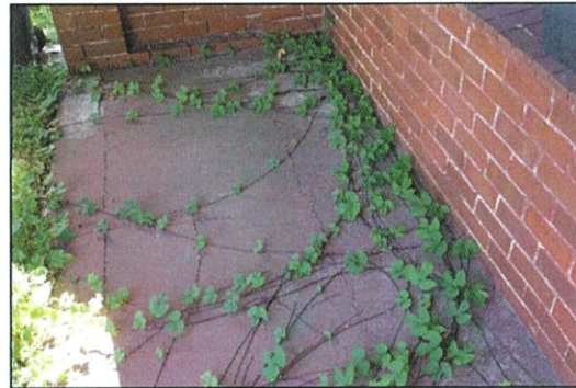
Figure 7. Close-up of painted concrete floor of verandah. Note creeping and self-seeded vegetation.
