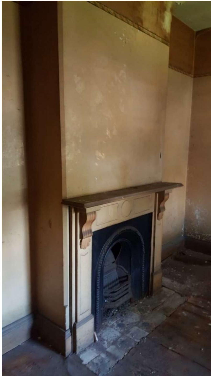
Figure 23 - Front western room showing existing fireplace with standard timber surround and cast iron register grate which are to be retained and conserved.
