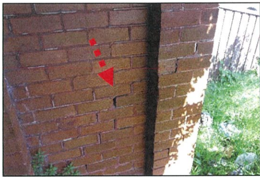
Figure 16. View to verandah blade wall. Note cracking, indicated by the red arrow.
