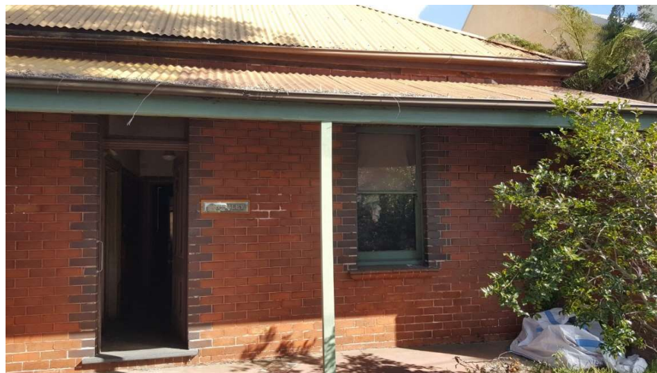
Figure 12 -Detail showing original name plate (Beverley), brick detailing and moulded brick sills, slate threshold and concrete verandah floor. The verandah beam is original and has a stop chamfered detail. The timber posts are modern replacements.
