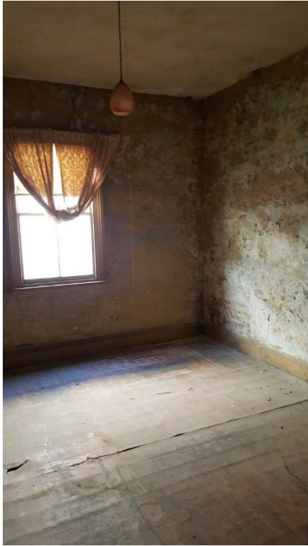
Figure 20 - Front room on eastern side (Bedroom) showing severely deteriorated plaster wall condition.
