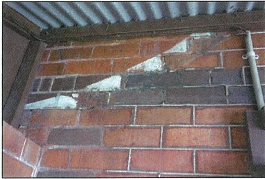
Figure 10. The faded outline, indicated by the red arrow, suggests that the current skillion form of the verandah is a later addition. The outline is present in the same location at both ends of the verandah.
