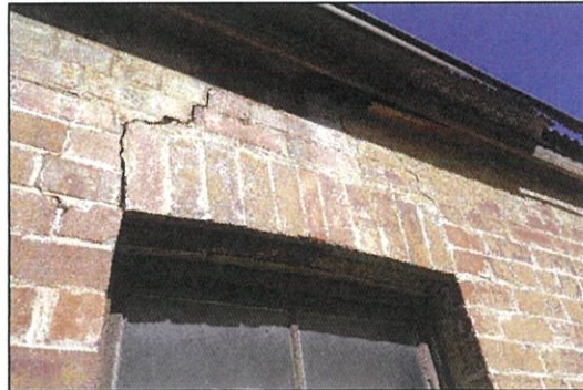
Figure 25. Close-up view of cracking, eastern elevation.
