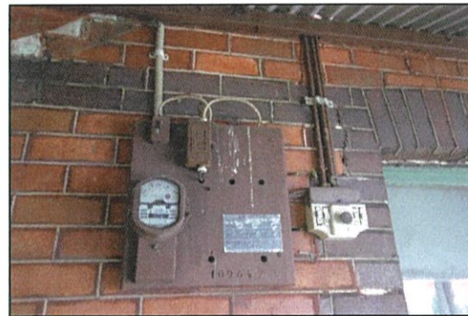
Figure 15. Close-up view of electrical board, northern elevation.
