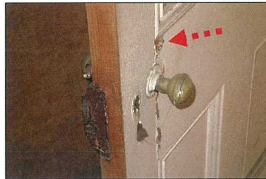
Figure 27. Close-up to D4. Note damage. Indicated by the red arrow.
