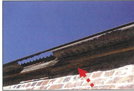
Figure 13. View to heavily Corroded gutter, eastern elevation. Note degradation to timber fascia, indicated by the red arrow.
