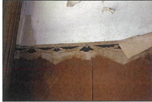
Figure 37. Close-up of wall paper at the dado, hallway.
