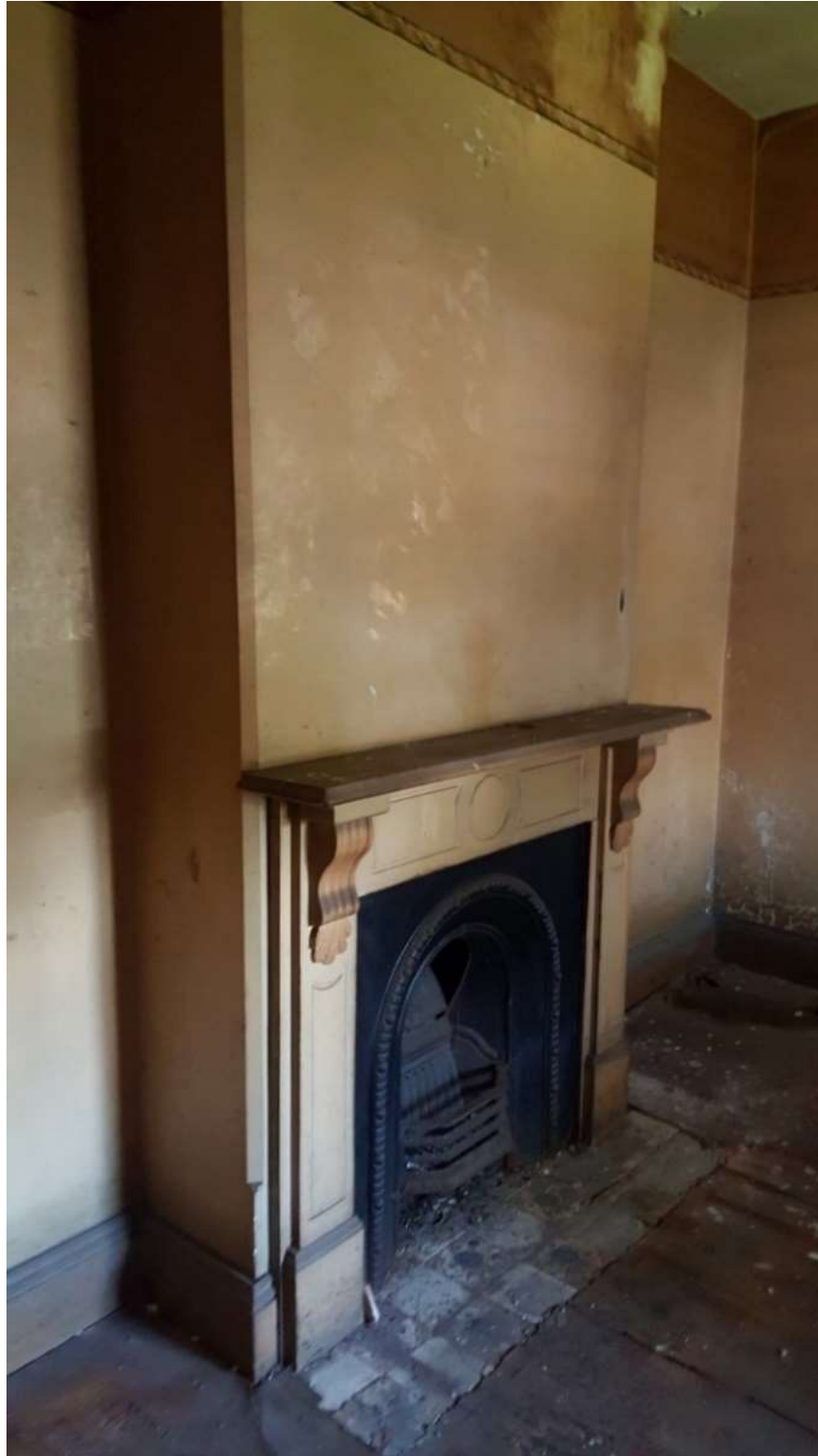
Figure 23 - Front western room showing existing fireplace with standard timber surround and cast iron register grate which are to be retained and conserved.
