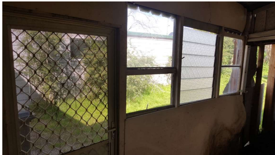
Figure 17 - Later fibro additions to rear of existing house enclosing covered access to kitchen and bathroom, proposed to be demolished.
